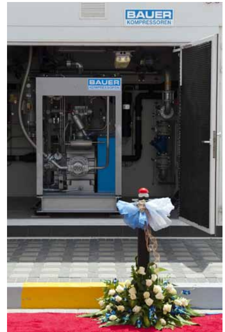
BAUER natural gas filling station in Abu Dhabi shortly before its inauguration.
