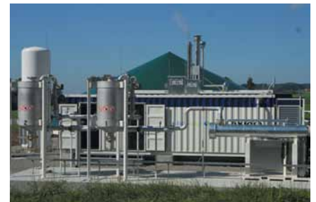
The Bebra biogas system.
